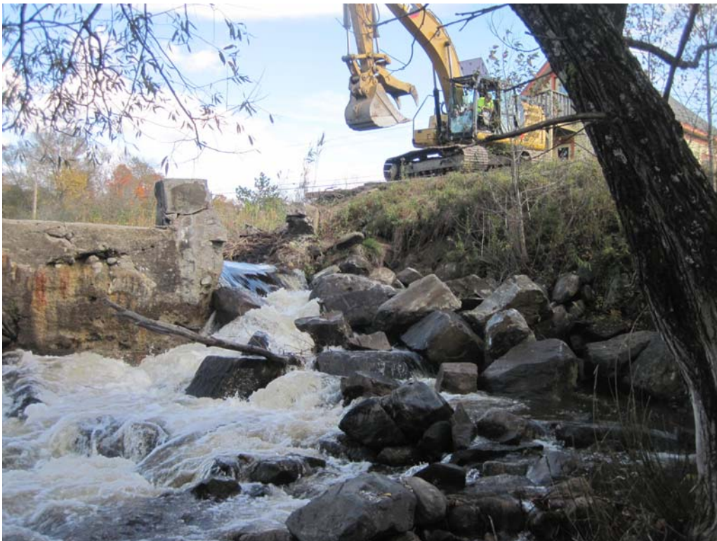
Armoring the eroded bank behind the Ice Cream Shop.
