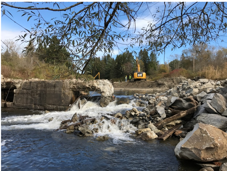
Breached dam and upstream sediment removal.
