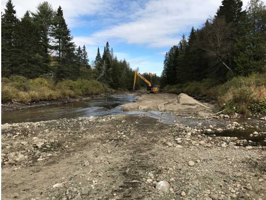
Initial sediment removal and haul road construction upstream of Dish Mill Brook.
