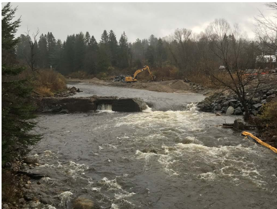
Partially removed dam under moderate flow. Scrap metal removal taking place in background.
