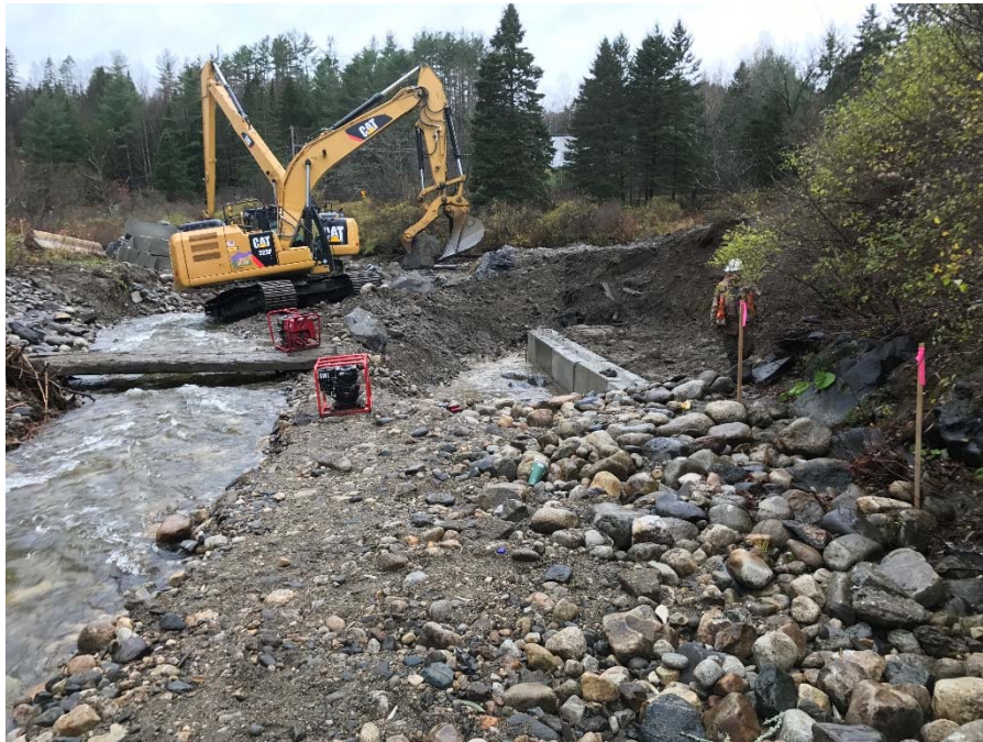
Installed base of right abutment and installation of bed armoring on Dish Mill Brook (looking downstream).
