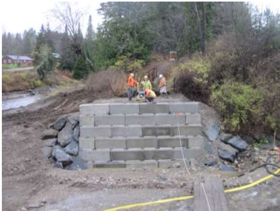
Completed right abutment on Dish Mill (looking from trail on left bank).
