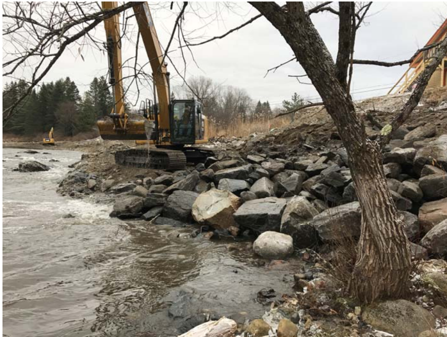
Shaped armor at bank erosion on river left at former dam site.
