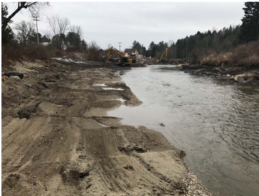
Excavated bench upstream of Dish Mill Brook. Sediment from channel to be placed on floodplain to build bar to proper elevation relative to channel.
